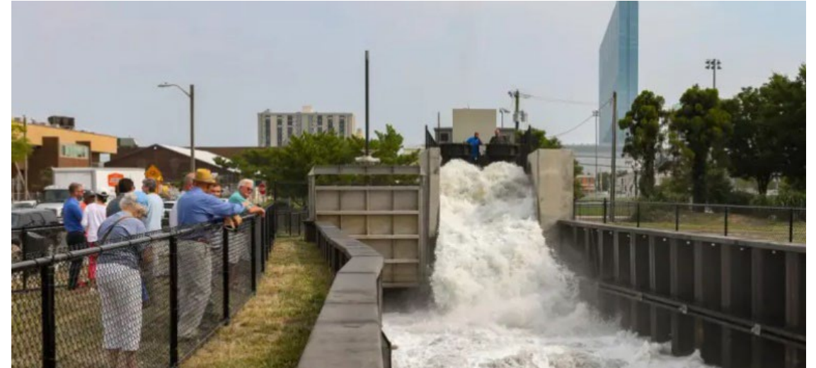
Recently installed pump station at Fisherman's Park Source: Press of Atlantic City, 2019
